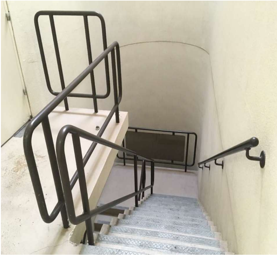
Non Compliant Stairway railings
