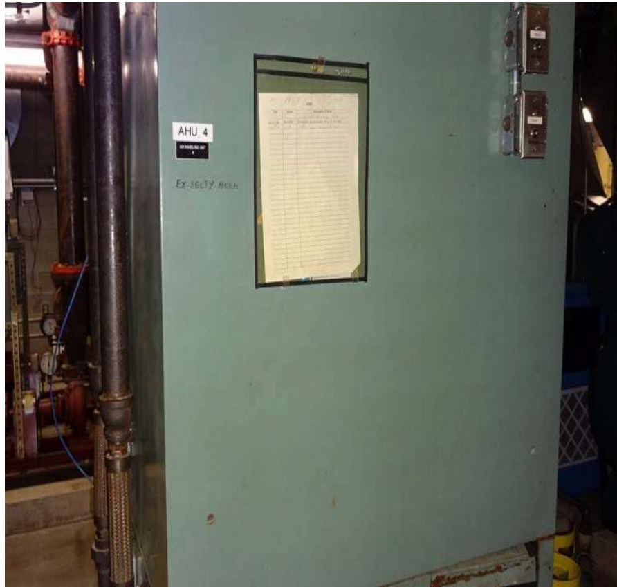
Original air handler - 1975
