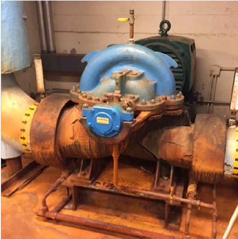
Failed Chilled Water Pump
