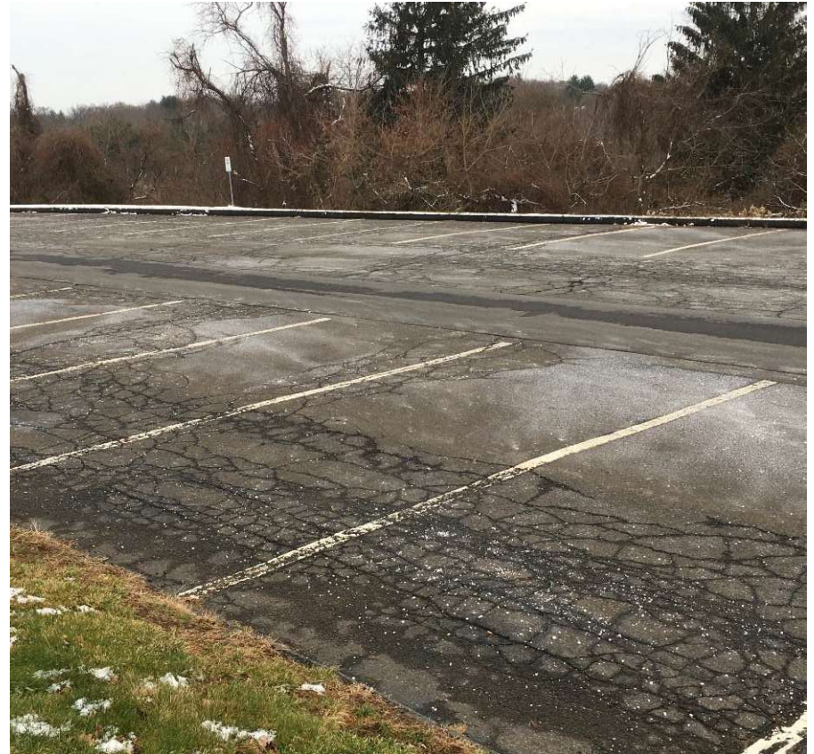
Failed Parking Lot Pavement
