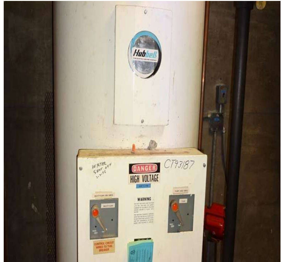
Original water heater – 1975
