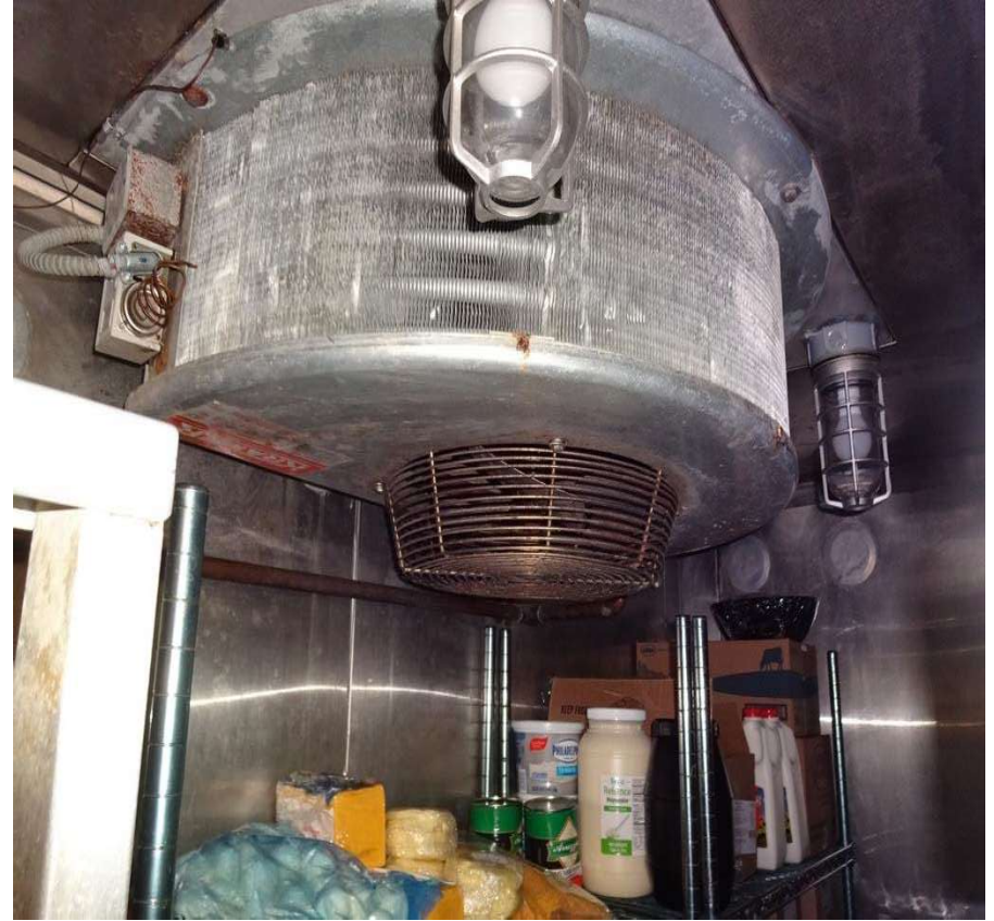
Old walk-in cooler and evaporative unit fan –
