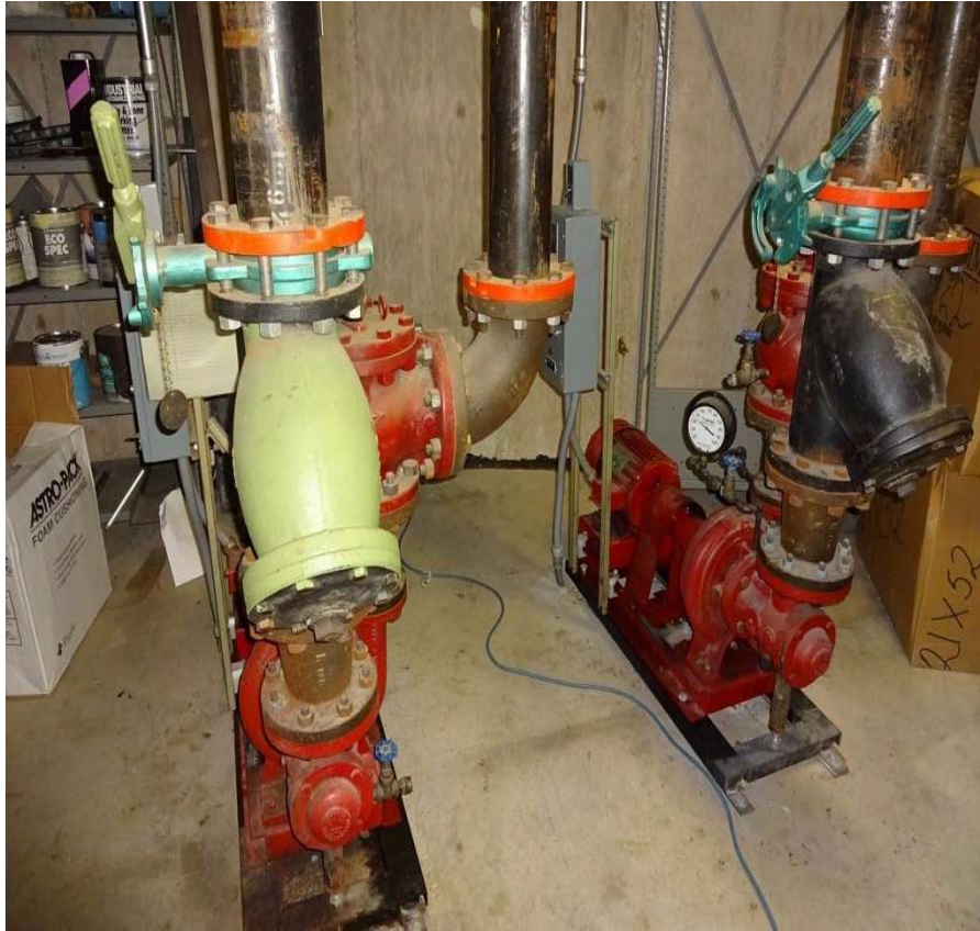
Aged and reworked hot water pumps
