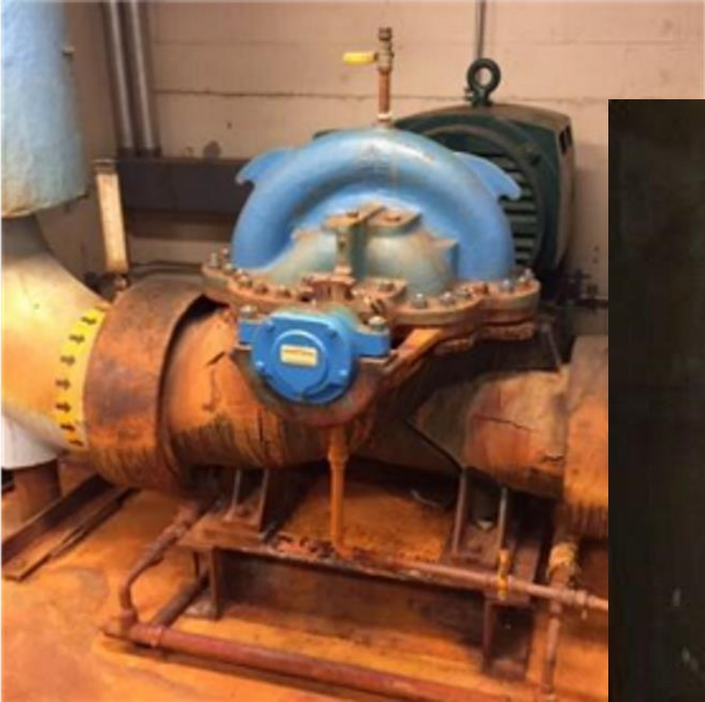
Failed Chilled Water Pump
