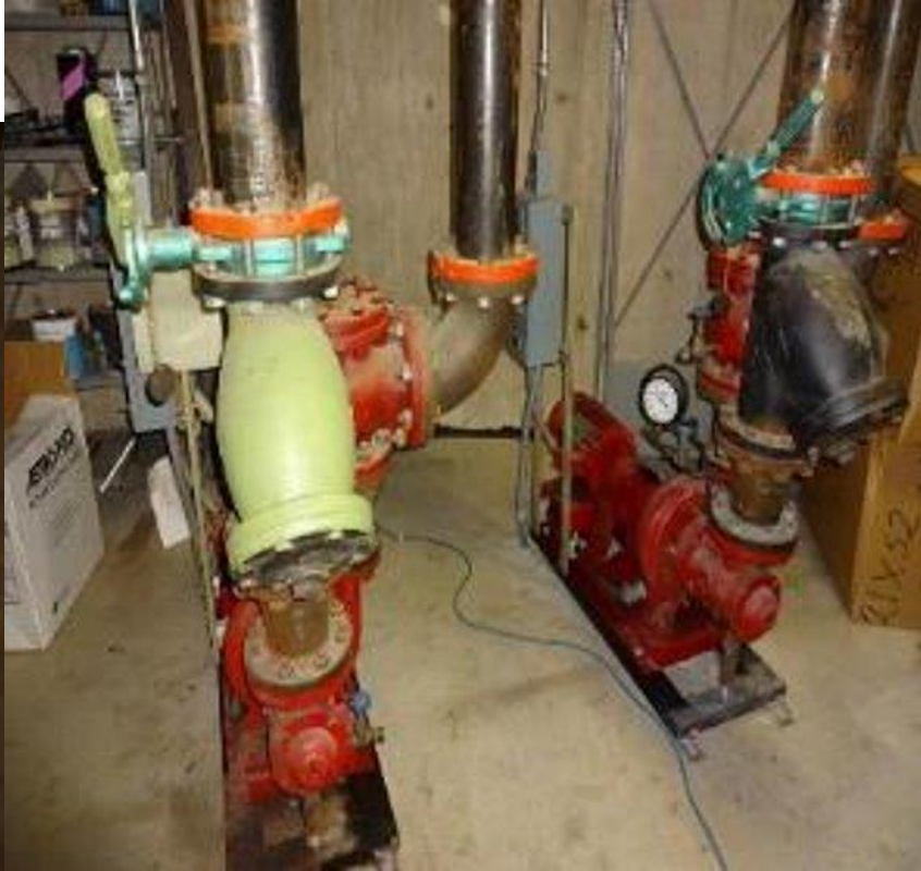
Aged & reworked hot water pumps
