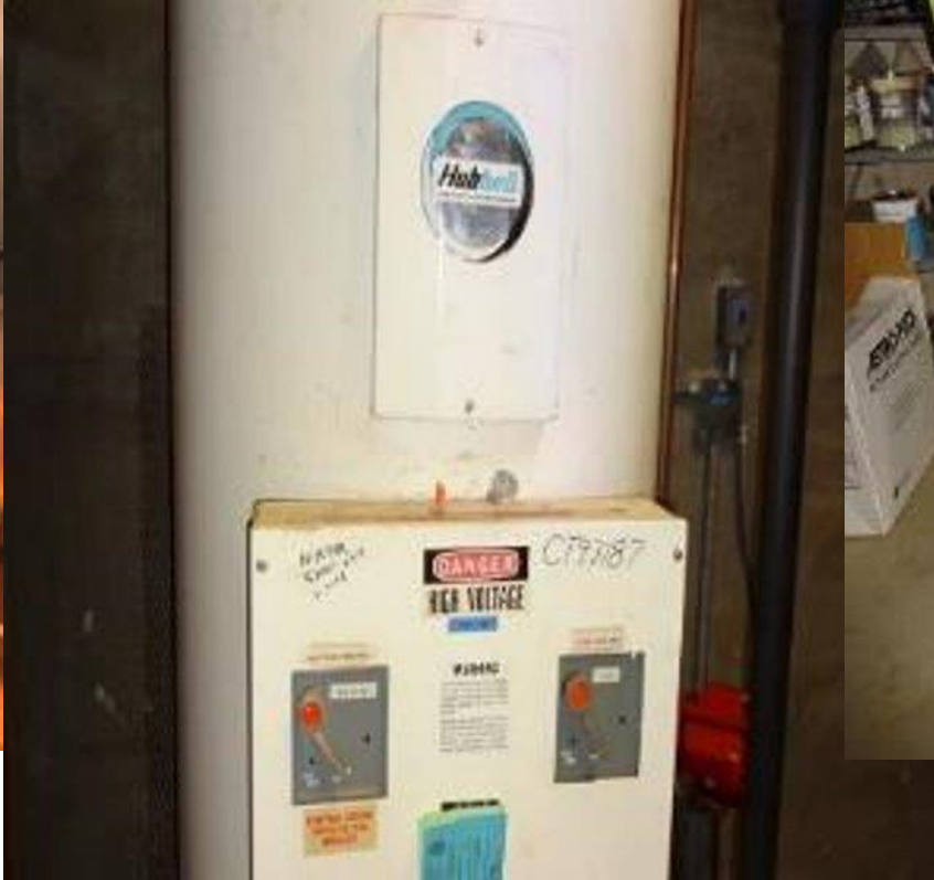
Original water heater – 1975
