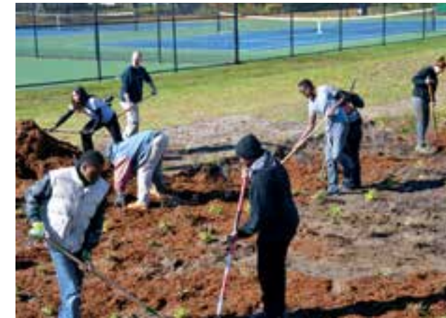
High school students work to install a rain garden as part of a UConn Natural Resources Conservation Academy initiative. (Contributed Photo)
