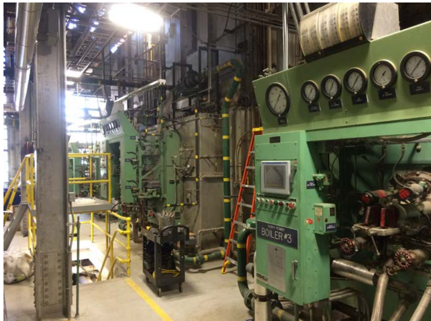
Existing CUP Steam Boiler 1 (1960), Boiler 2 (1962) and Boiler 3 (1966)
