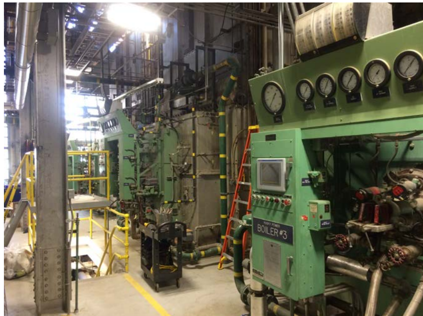
Existing CUP Steam Boiler 1 (1960), Boiler 2 (1962) and Boiler 3 (1966)
